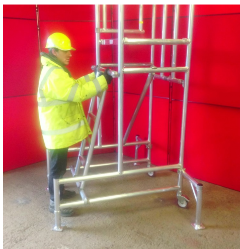
5) CLIP UPPER BRACE OF LADDER ABOVE RINGS ON VERTICALS WITH ASSEMBLED HOOKS ON TOP
